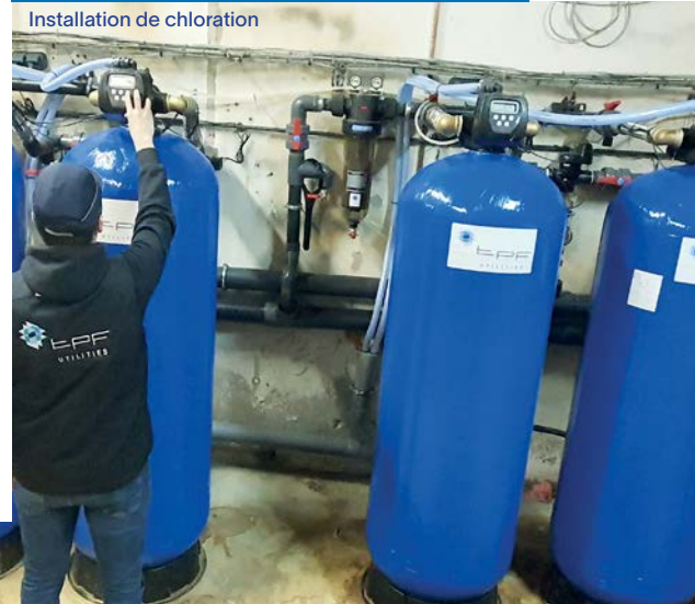
Installation de chloration
