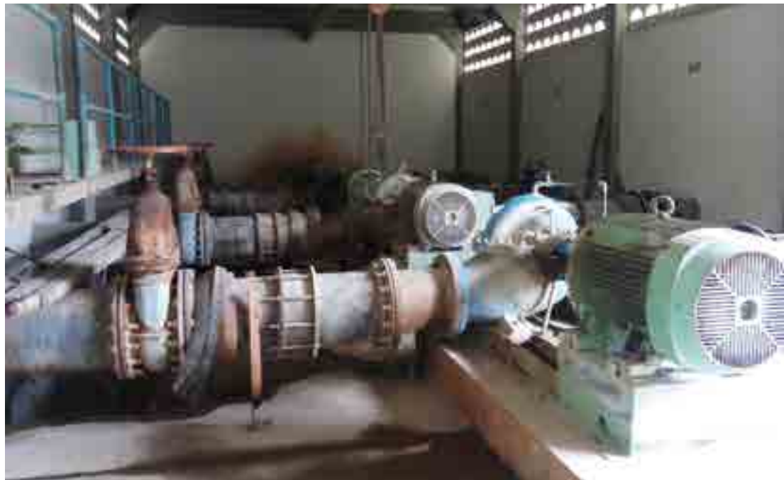
Automation of pumping systems in irrigated perimeters
