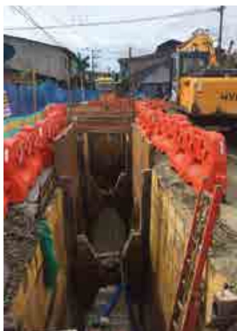
Sewer collectors in Quibdó
