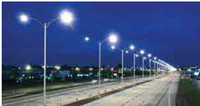
Modernization of public lighting in the Walloon Region
