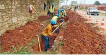
Uíge water distribution network / Angola
