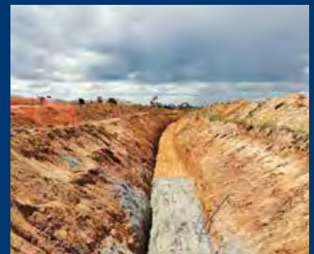
^ Water supply system of Morgável
