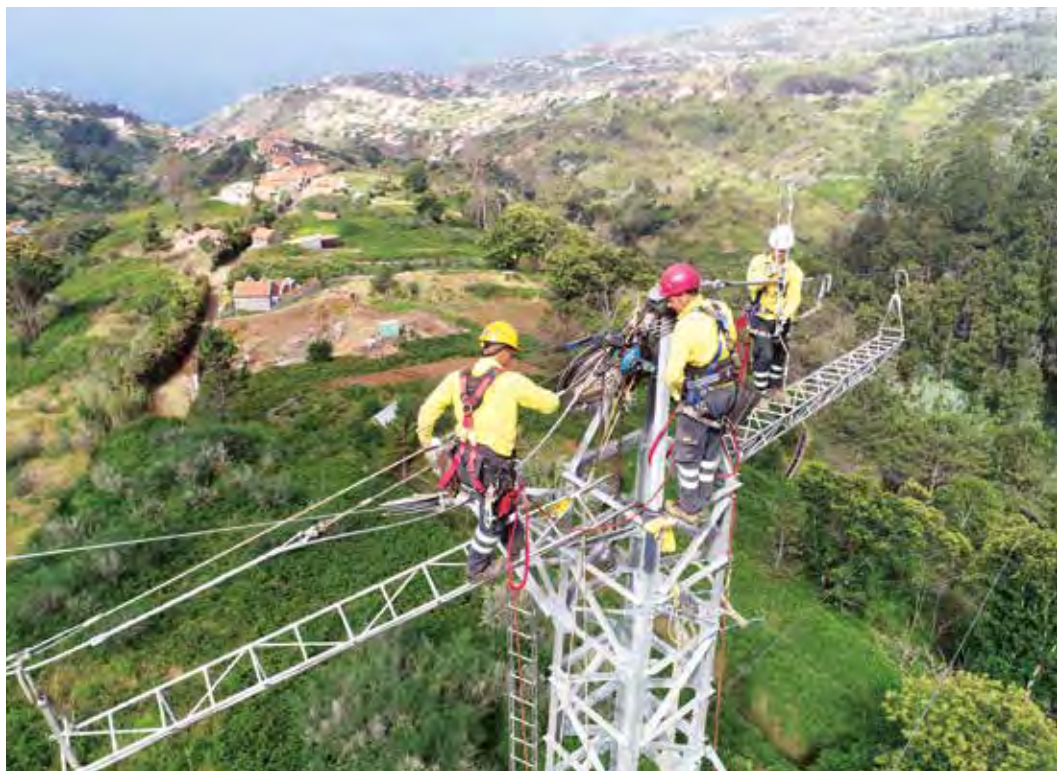
> Calheta hydroelectric project
